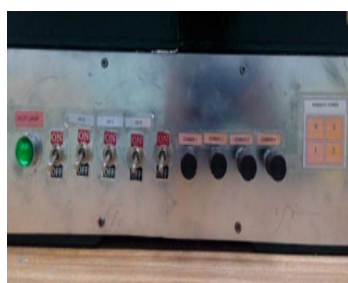
Figure 6. Control Panel of the Reactor
